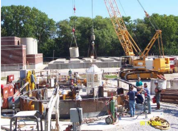
A bustle of construction activity at an access shaft within a pristine park setting
