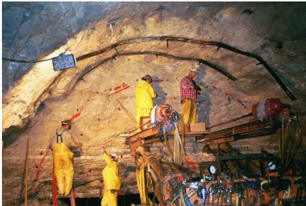
Workers prepare for explosive charges to blast bedrock out of an access shaft.
